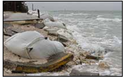
Eroded parking lot
